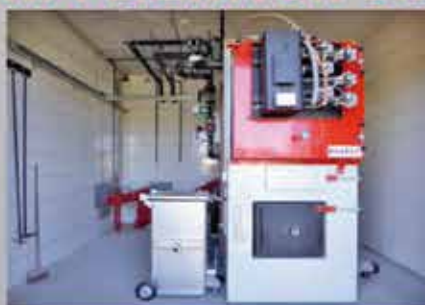
District heating plant HPKI-R 300
