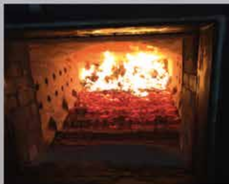
Fire brick lined combustion chamber with moving step grate
