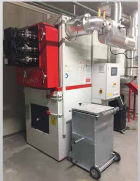
Side mounted control panel
