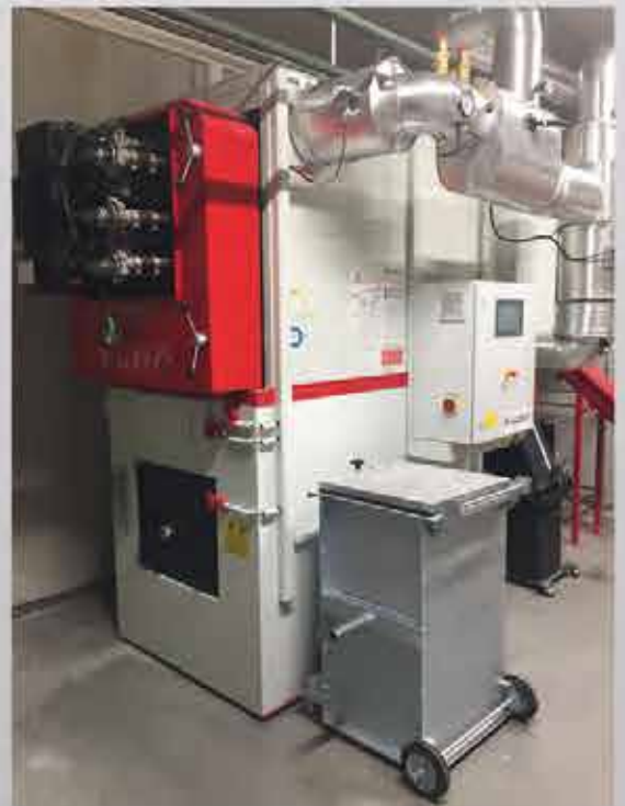
Side mounted control panel
